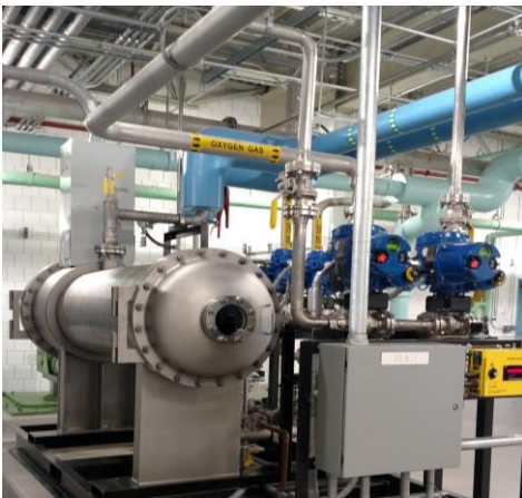
New Ozone System installed in 2017 at CLCJAWA
